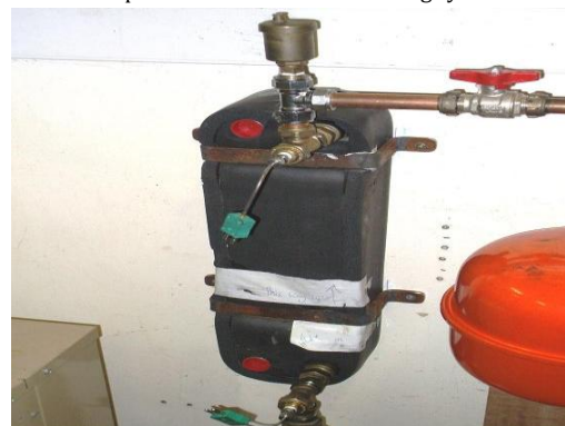
Figure 14: Shows the heat exchanger
